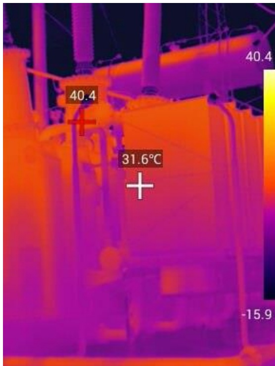
Fig.5. AT radiator thermogram
