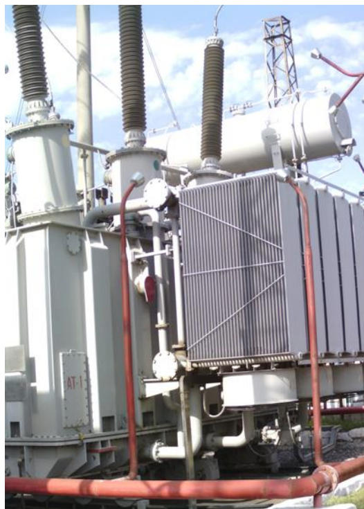
Fig.6. The appearance of the radiator AT
